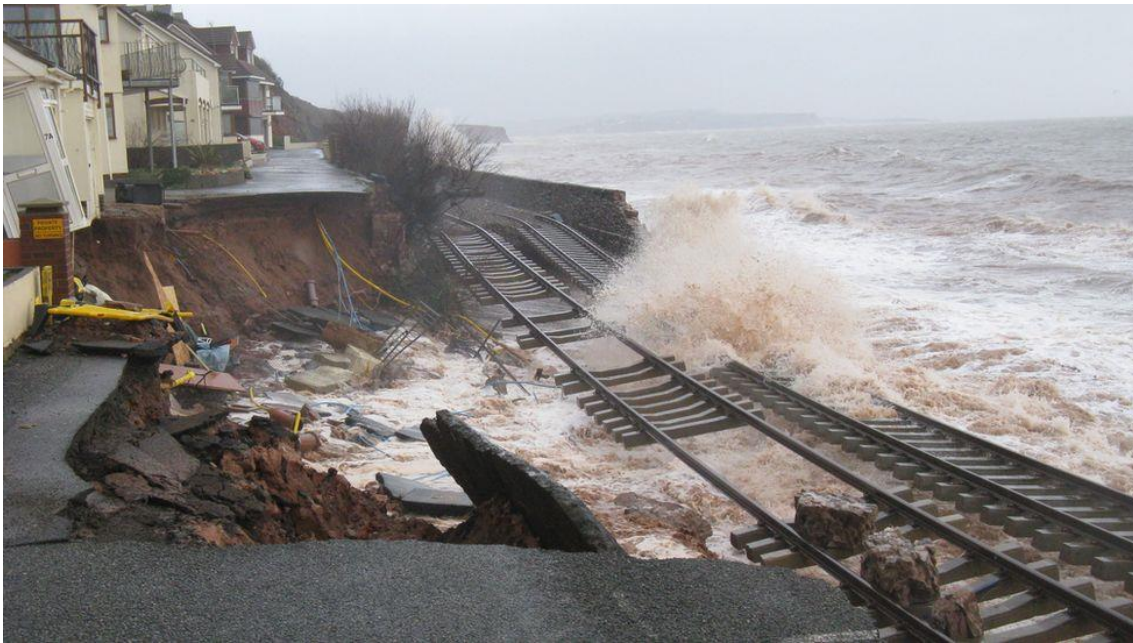
Figure 6: Significant damage to the rail network at Dawlish following the 2014 storms
