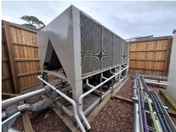
Figure 1: Heat pump system at Newton Abbot Leisure Centre.
