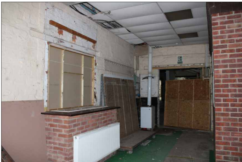
Plate 11: Internal view of structure 4, showing blocked openings in the north wall, looking north
