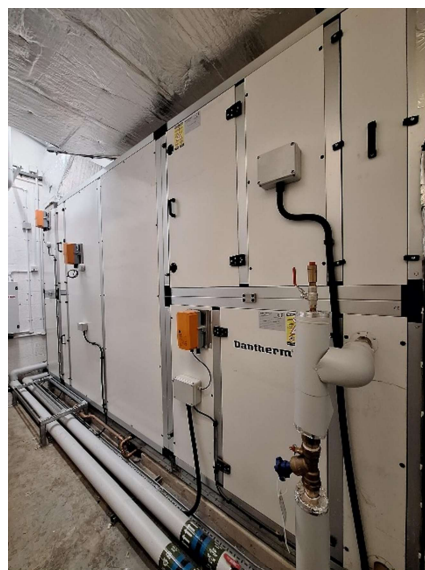
Figure 6: New high-efficiency ventilation system at Dawlish Leisure Centre.
