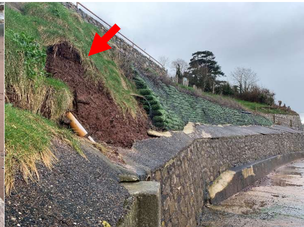
No AIMS Asset ID Erosion of grass bank as southern end of wall.
