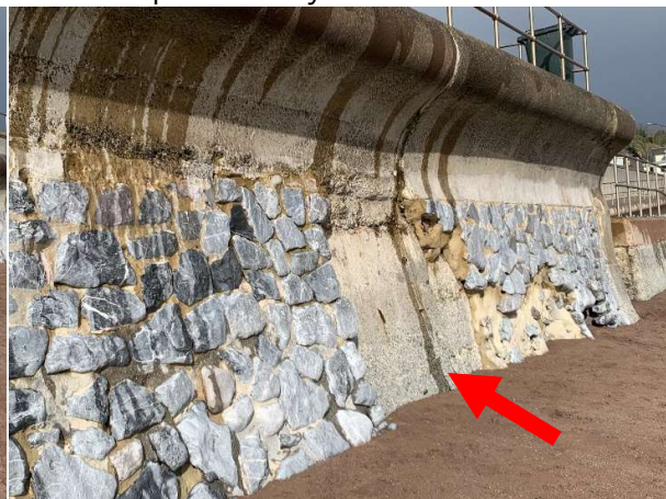
177501 Localised loss of section of masonry facing at northern end of wall exposing concrete backing.
