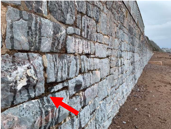
No AIMS Asset ID. Masonry blocks sound, minor abrasion to mortar joints.
