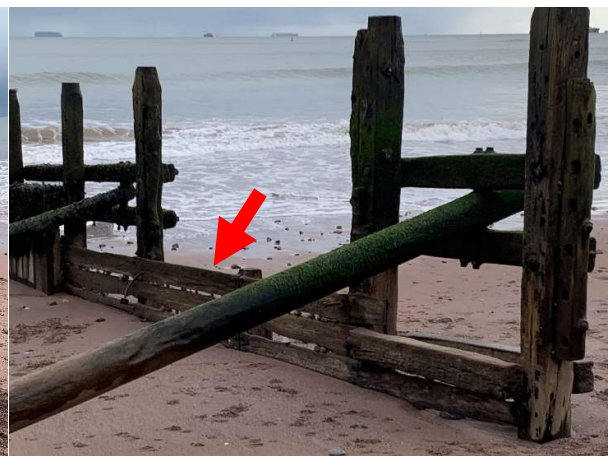
327117 Heavy abrasion of posts and planks with gaps showing between boards.
