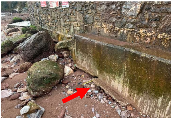
84537 Low beach levels at southern end of wall near outfall resulting in localised undermining up to 0.9m deep.
