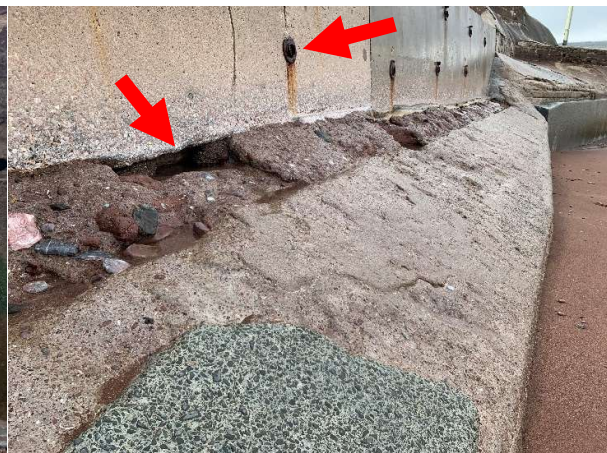
No AIMS Asset ID Heavy abrasion and voids opening in toe. Most flap valves missing.
