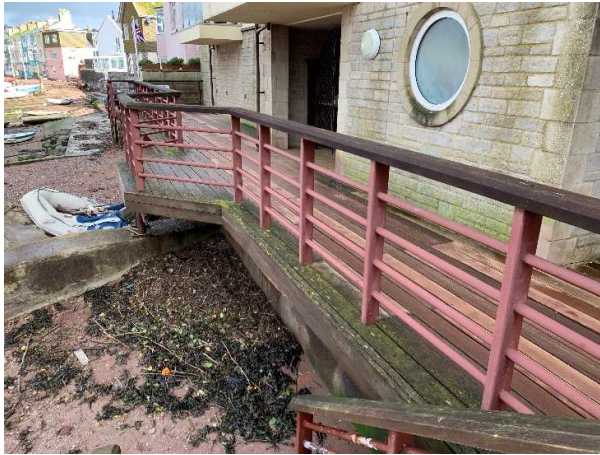
3934 No gaps or damage to timber boards or hand railings along crest of concrete wall.
