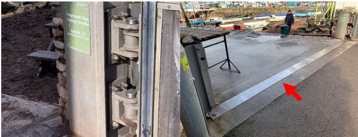
392735 No corrosion to hinges which appear to be in good working order.
