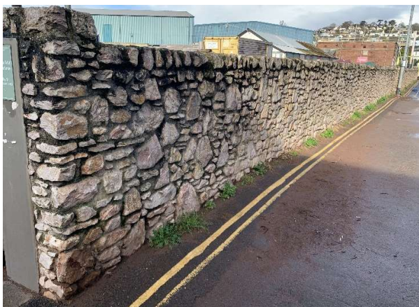
180688 No gaps or cracks in masonry or mortar joints in new walls constructed.
