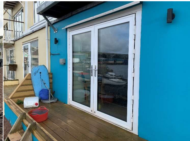
42304 All flood proof doors to property defence line along back of beach in good condition.
