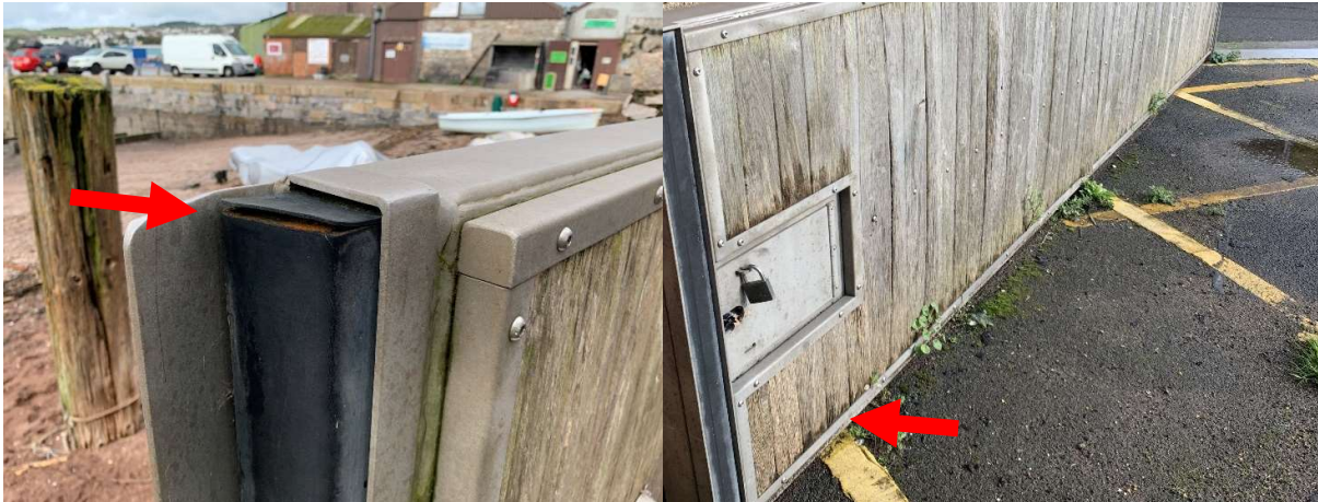
392754 Minor cracking evident to most rubber seals, with some delamination of one seal (flood gate No.12).
