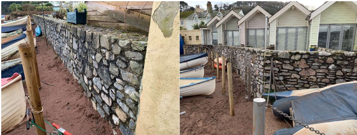
82711 Masonry blocks in good condition, no cracking or gaps in mortar joints, all flap valves present and working. 82719 Masonry blocks in good condition, no cracking or gaps in mortar joints, all flap valves present.
