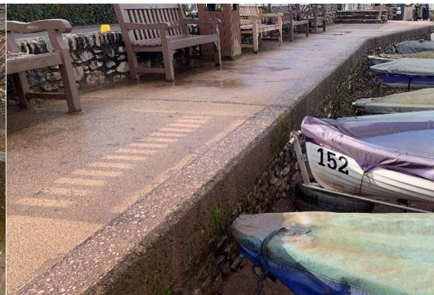
84537 High beach levels along promenade, concrete surfacing and masonry setback wall in good condition.
