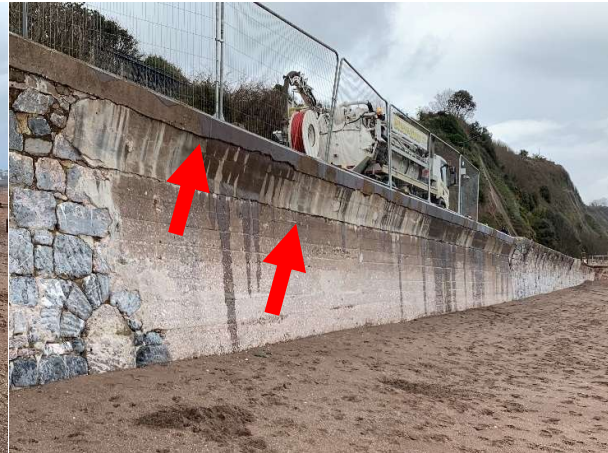
No AIMS Asset ID. Small horizontal cracks between construction joints at repaired section of wall.
