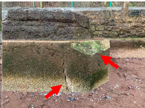
84539 Abrasion along concrete toe and localised cracks and missing sections of some concrete.
