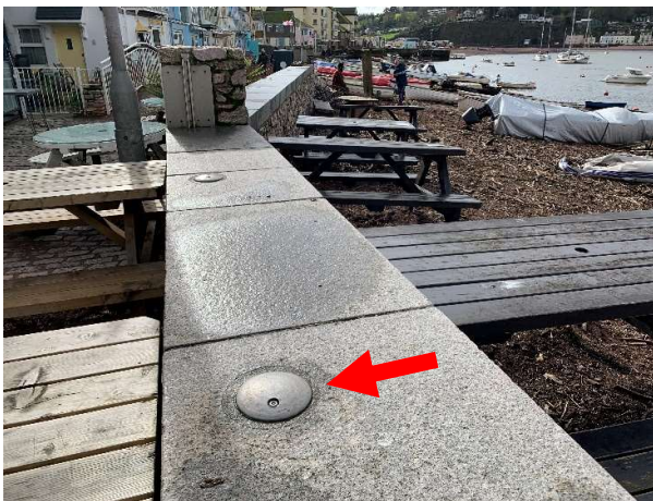
524451 All post caps and hold down bolts present and in very good condition.
