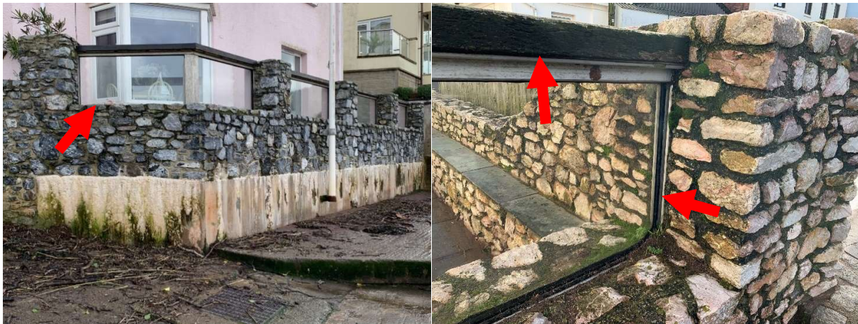
392781 Waterproof glazing panels in good condition. 392781 Seals to floodproof glazing panels intact. Some rot evident in lintles.
