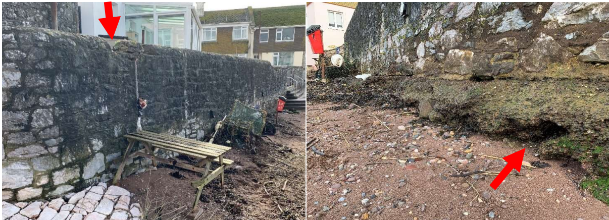
392776 Masonry blocks and mortar joints good, two short sections of missing coping stones.
