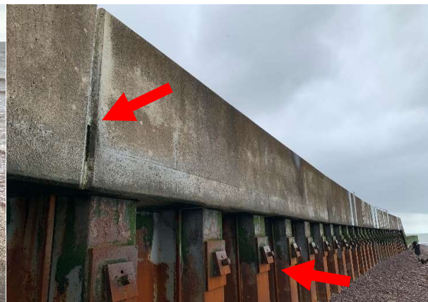
57776 Loss of paint system and surface corrosion of toe piles. Loss of majority expansion joint sealant.
