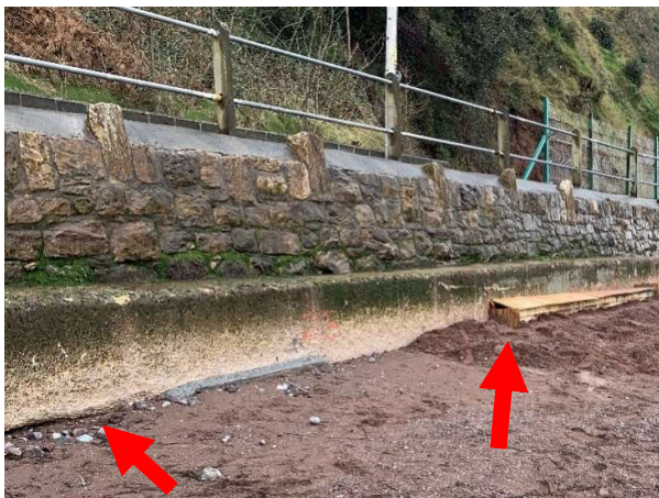
84539 Evidence of undermining of concrete toe, concrete fill repairs underway at time of inspection.
