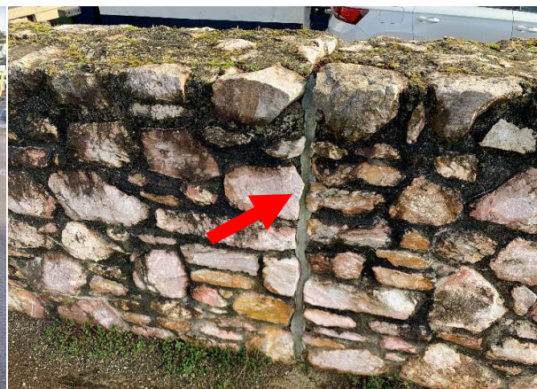
180688 Joint sealant in new masonry walls remains in good condition with no signs of debonding or cracking.
