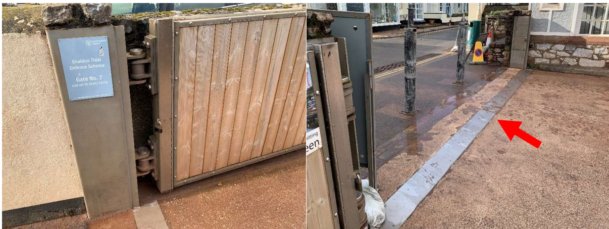
332933 No corrosion to hinges, all appear to be in good working order.
