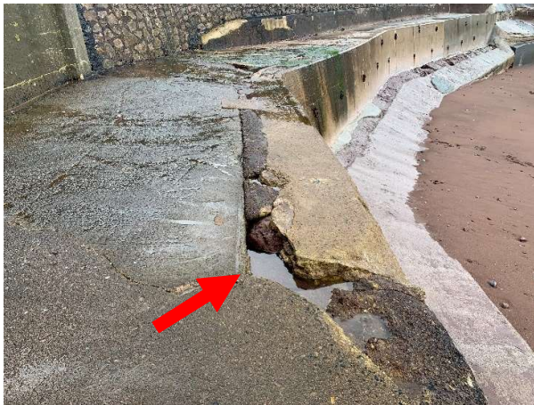
No AIMS Asset ID Cracks in concrete and rendering, some sections of concrete broken and missing.
