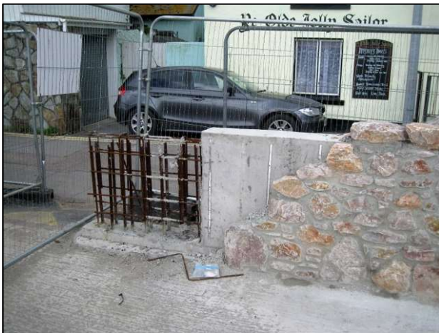
Figure 2.16 Construction of reinforced concrete floodwalls with masonry facing as part of the Teignmouth flood defence scheme (R. Scott 2012).
