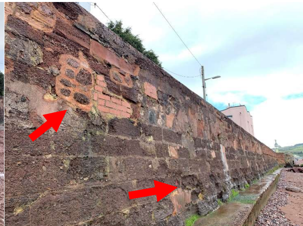
84538 Heavy abrasion to masonry blocks along some sections of wall, especially at toe, many brickwork repairs but in reasonable condition.
