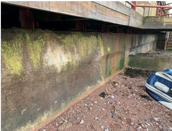
3934 Minor cracks evident in concrete wall but render largely intact along northern end.
