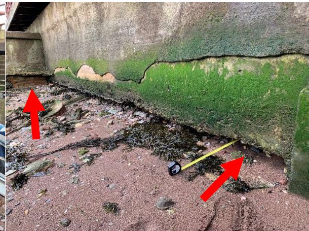
3934 Some cracking and spalling evident in concrete render, beach lowering and localised undermining of toe.
