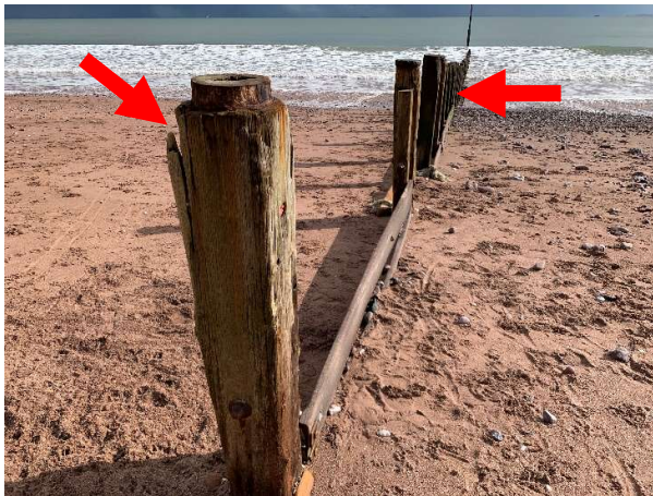
327084 Most posts vertical with only minor rotation evident. Many posts split and cracked.
