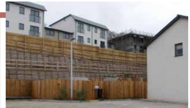
Poor handling of level changes
